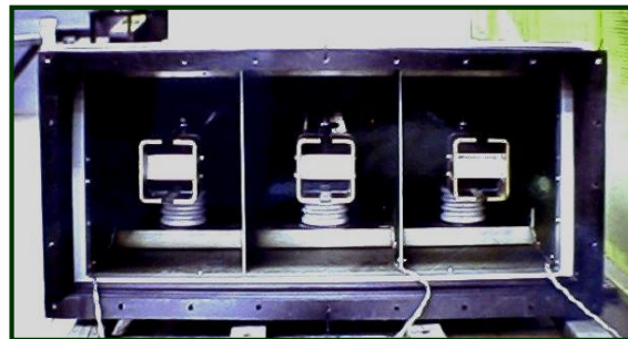
Segregated Phase Bus
